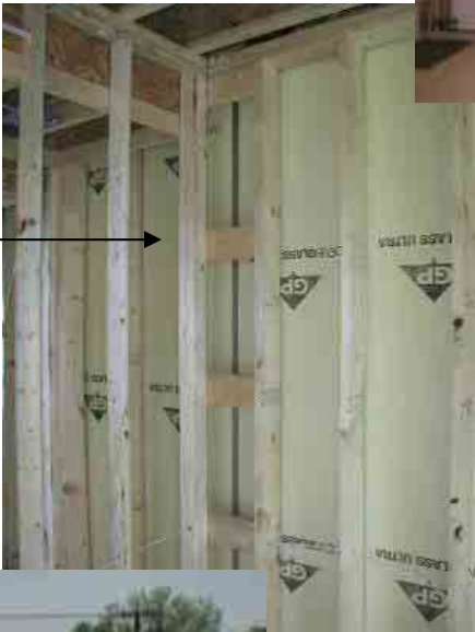
Advanced framing techniques like this ladder corner allow better insulation and save wood resources.
